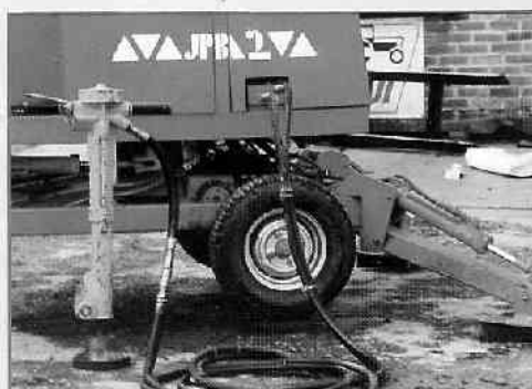
Power breaker plugged in and ready for operation
