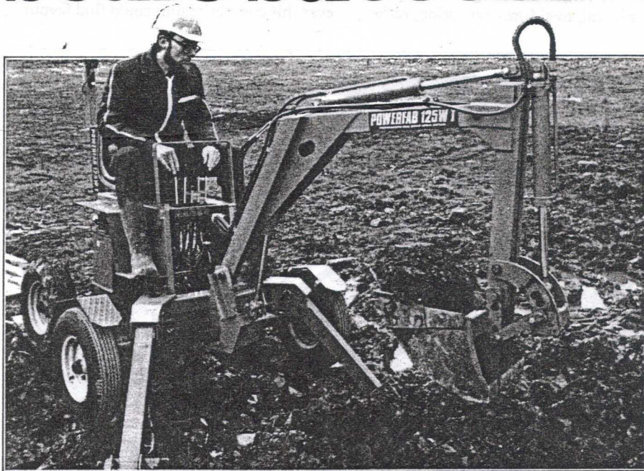
Nick Johnson at the controls to remove another bucketful of Welsh muck.
